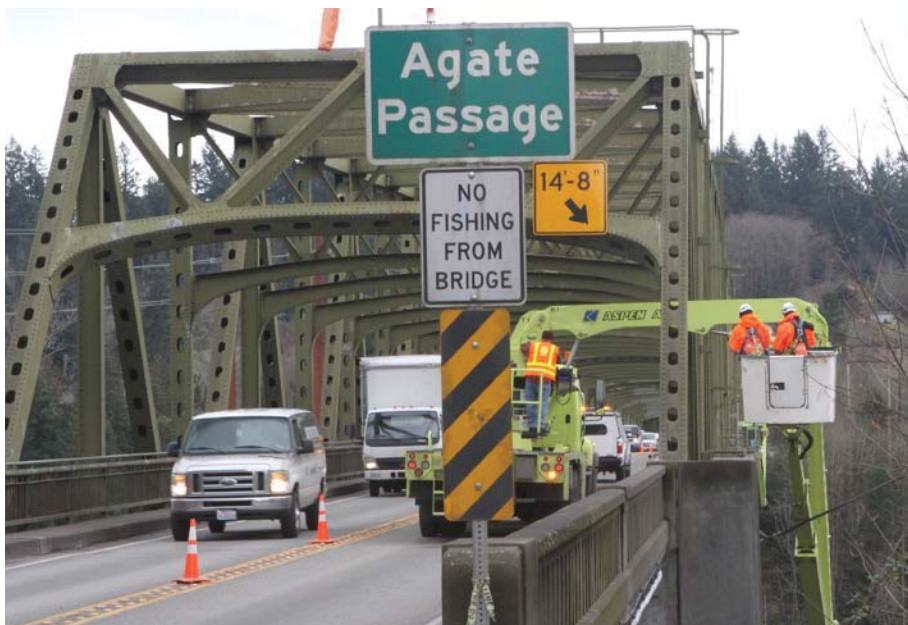
WSDOT conducted maintenance/washing activities on the State Route 305 Agate Pass bridge between Suquamish and Bainbridge Island in February 2017.
