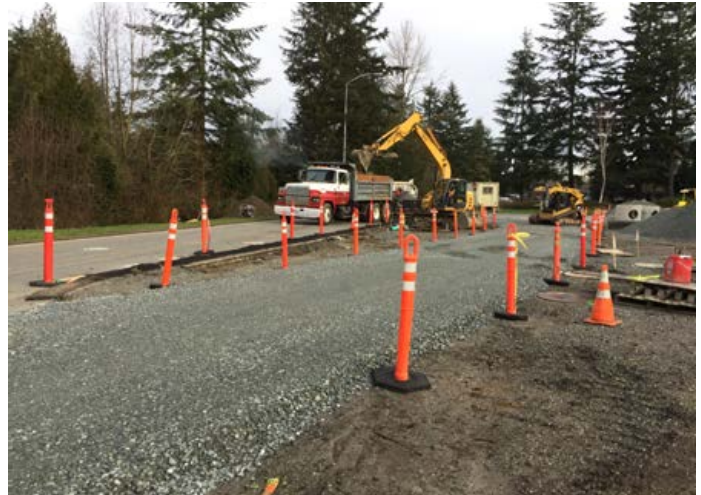
Renovations to winterize and replace components at the Silverlake rest area off Interstate 5 near Everett began in February 2017.
